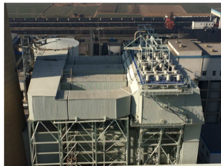
Figure 5. Wet ESPs for 660 MW unit Hebei Guohua Dingzhou Power Generation Co., Ltd.
