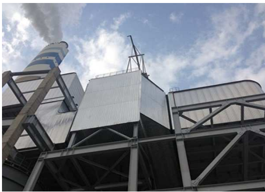
Figures 4. The actual picture of WESP used in Shanghai Caojing 1000 MW coal-fired power plant
