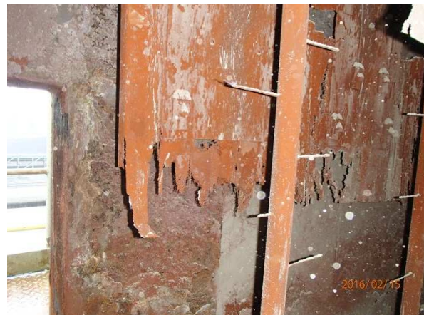
Figure 1. Corroded collecting plates on the way of colder gas flow in the ESP
