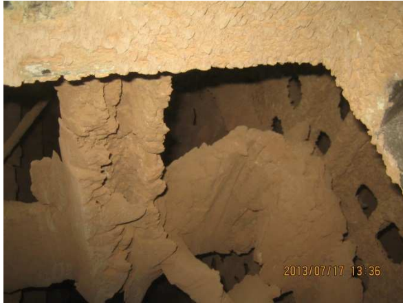
Figure 4. Hard dust build –ups on stiffeners of ESP of the flash copper smelter
