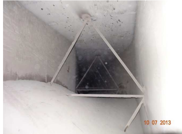
Figure 3. Dust build-ups in oversized gas duct before the ESP
