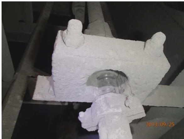
Figure 2. Fast wear of rapping shaft and hardened bearing on the way of colder gas flow in the ESP
